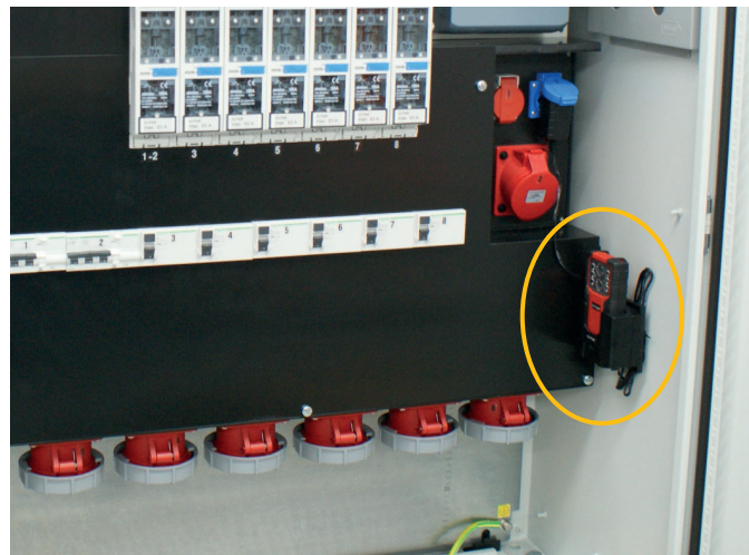
TorchLED Emergency in a construction site cabinet
